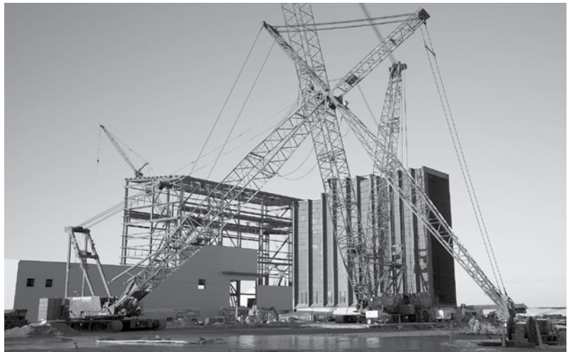
Above: Natural gas power plants, like Deer Creek Station under construction by Basin Electric Power Cooperative, are likely to fulfill our electricity needs in the short-term. Opposite Page: Tri-State Generation & Transmission Association, based in Colorado, is part of one of the largest solar projects in the nation, the Cimarron Solar Facility in New Mexico. Solar-powered generation is becoming more popular as states set renewable energy standards. Source: Tri-State Generation & Transmission Association
