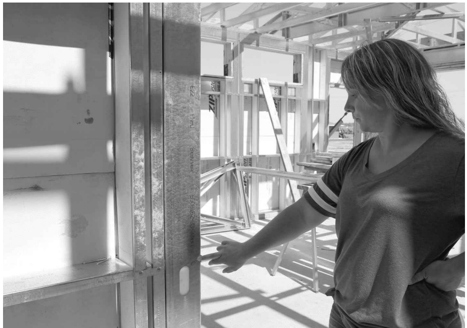
Jackie Adolph points to a label on one of the steel components, which was generated by the design software to ensure the pieces are properly assembled. Photo by Shannon Marvel
